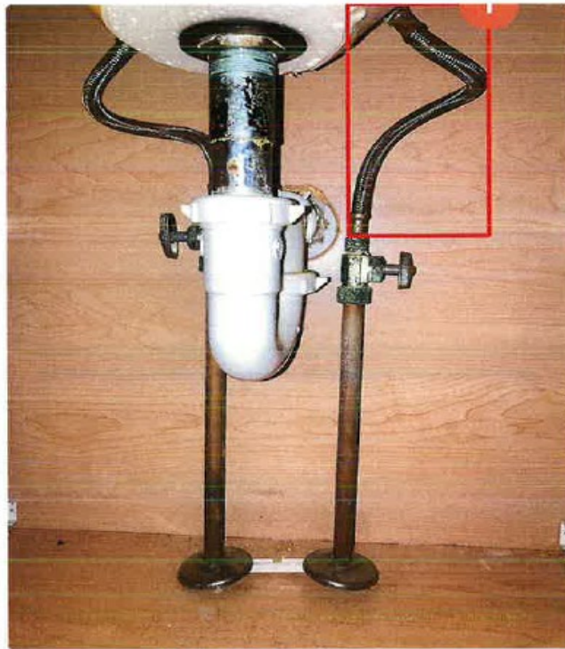
Bathroom 2 > Sink Plumbing 2
